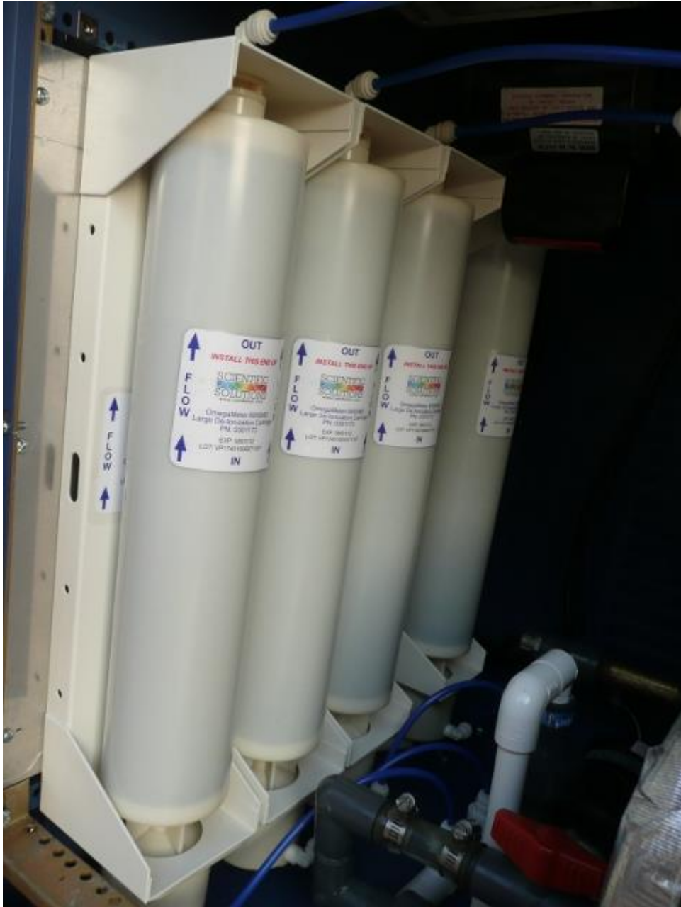
Quick-Disconnect D.I. Columns mounted in cabinet
